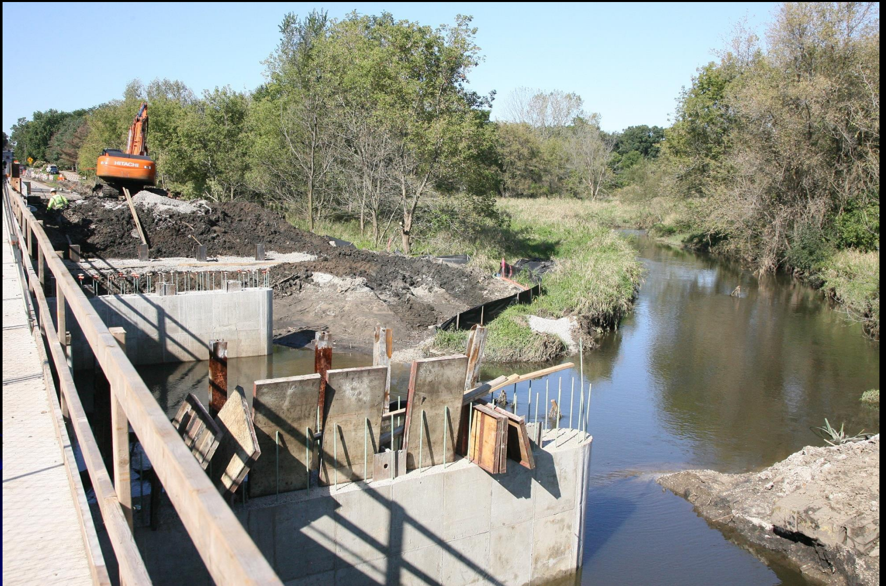
Crews continue to frame and pour support columns for the north half of the new bridge on the Silver Glen over Otter Creek bridge replacement project
