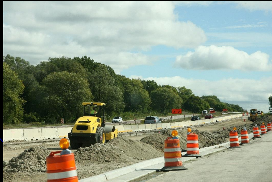
Crews continue to grade for the new ramp and construct the new MSE wall as part of the Randall Road at Weld Road/US 20 intersection improvement project
