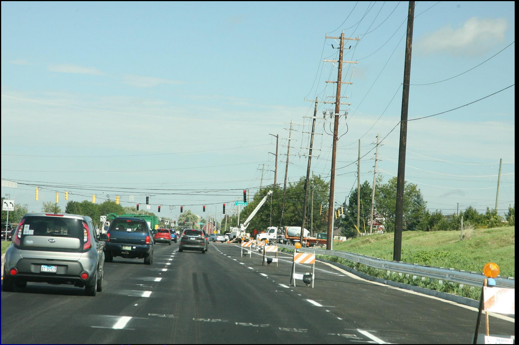
New striping, wearing surface course and guardrail give the roadway a new look as the project moves to traffic signal work on Randall Road as part of the Stearns Road at Randall Road intersection improvement project
