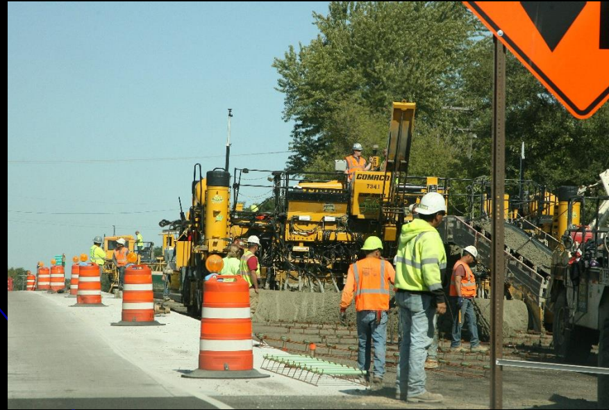
Crews pave the new portion of Longmeadow Parkway between IL route 25 and IL route 62 as part of the LMP Section C-3 IL 25 Intersection Improvement project
