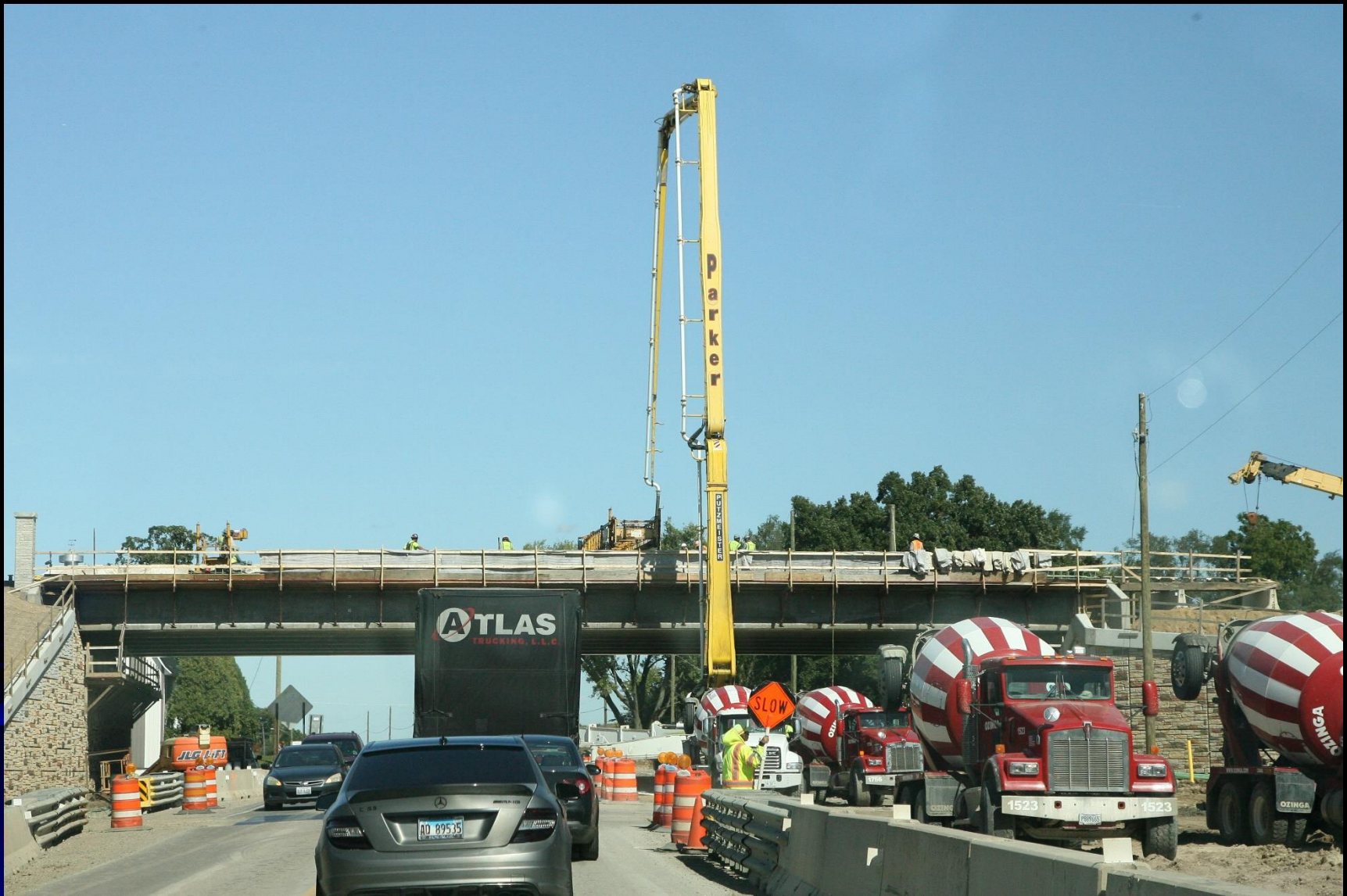
Crews pour the deck for the new bridge over IL 31 on the LMP Section B-2 contract
