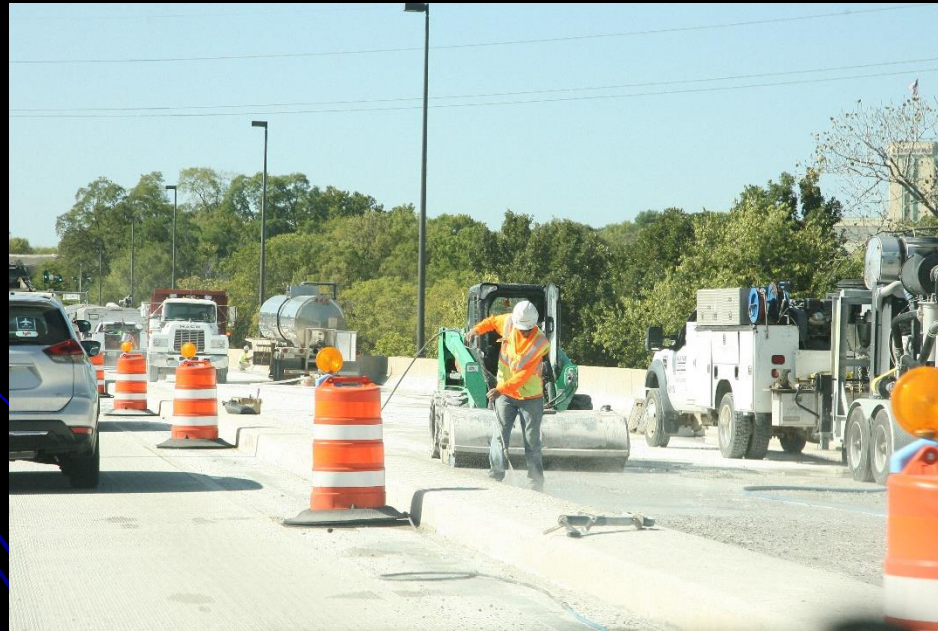
Crews resume hydro demolition on the bridge for the Fabyan over Fox River Bridge improvement project
