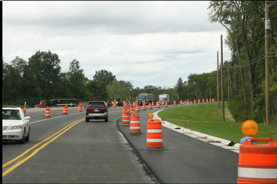
Crews place surface course for the new roadway on IL 62 as part of the LMP Section D – E/O IL 25 to IL 62 contract
